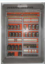
Hydro Pumping Panel
