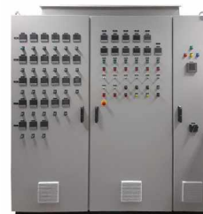
Crusher Plant Panel
