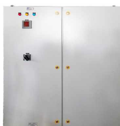
Solar ACDB/DCDB Panel
